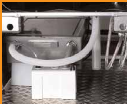
Clean the siphon, neutralisation unit and condensate pump
